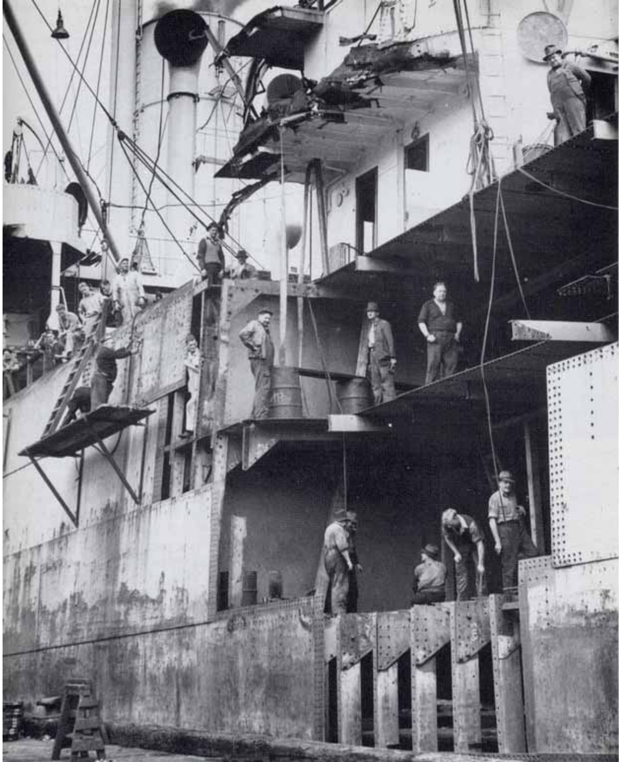
Workers in the dry dock at Cockatoo Island replaced a large hull section on SS Clan Chatton in 1945. From Rosemary Broomham, Steady Revolutions; The Australian Institute of Marine and Power Engineers 1881-1990 , Private Collection
